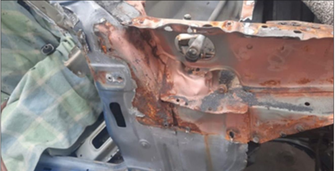
Image 1: In this photograph, the copper-based primer chosen and applied during a previous repair is inappropriate, and as a result, its presence has not only failed to provide the corrosion prevention expected of it by the repairer, but has in fact promoted further corrosion on the vehicle's structure.
