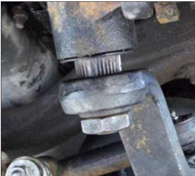
Image 30: Very little of the sector shaft is visible for inspection.
