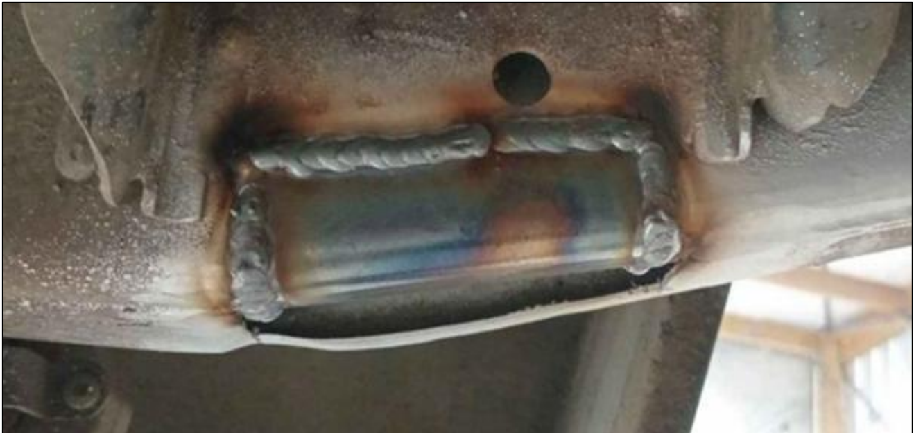
Image 5: Typical example of a conventional corrosion damage welding repair being performed on a chassis rail which has a tensile strength of 440 MPa or less.
